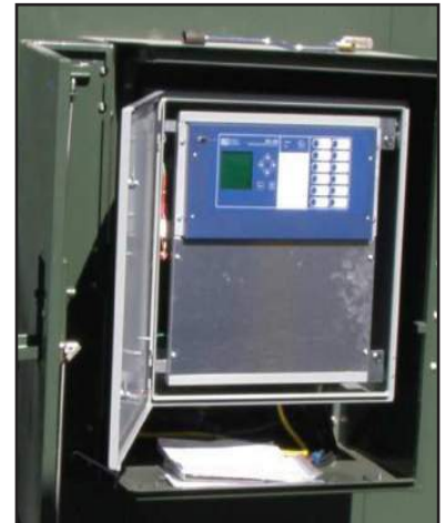
Control located on automated Trident
