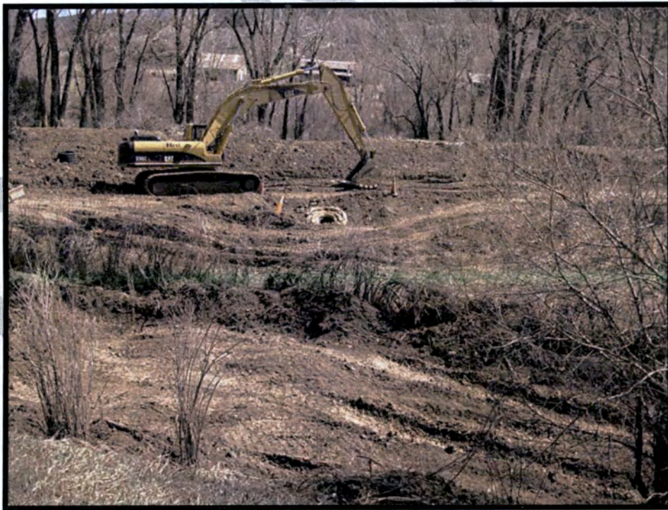
Photo 15. Table 4, Unit 1; Table 1, Unit 10. Same wetland as in Photos 12, 13, and 14 showing the drain in wetland. A drain was placed in the wetland, draining the wetland into the irrigation pipe further impacting the wetland
