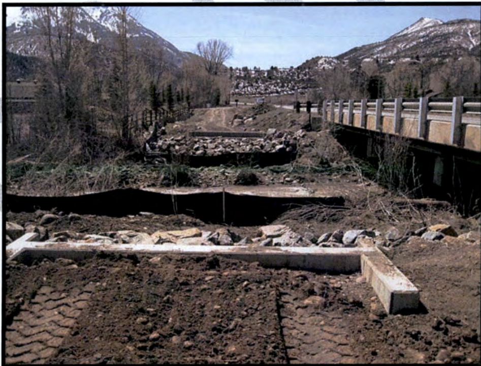
Photo 11. Table 1, Unit 9. (EES wetland report Figure 12). Photo taken north to south which shows bridge abutments and disturbance with this activity.
