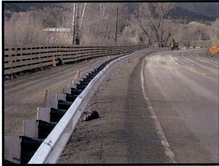
Photo 30. Dead raccoon along road at guard rail and wildlife barrier fence. Wildlife mortality in this reach will probably rise since there is now over 2,044' of wood fence and elevated trail and bridges in a continuous stretch beginning at Prince Creek and continuing to the south side of the Hwy 133 Bridge across the Crystal River. There is a 200' section woven wire fence that is low enough for deer to jump over, but no gap on the bottom to allow young deer or other wildlife to pass under. A raccoon could go under the wood fence, but all this infrastructure probably adds to the confusion of animals already stressed trying to cross the highway. This will cause increased exposure time between wildlife and increase vehicle accidents.
