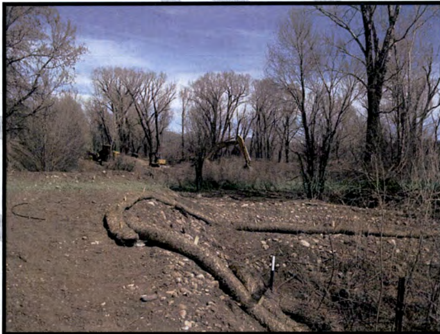
Photo 13. Table 4, Units 1 and 2; Table 1, Unit 10; (EES wetland report Figure 10). The wetland is 0.47 acre at north end of field. Extensive excavation was done in the wetland to create the trail and install irrigation pipe to replace the ditch. Although replacing the ditch with a pipeline is a more efficient way to transport water for agriculture it dewateres the wetland that was previously recharged by the ditch. Wetland habitats are very limited in the lower Crystal River Valley; the few wetlands that exist provide valuable wildlife habitat.
